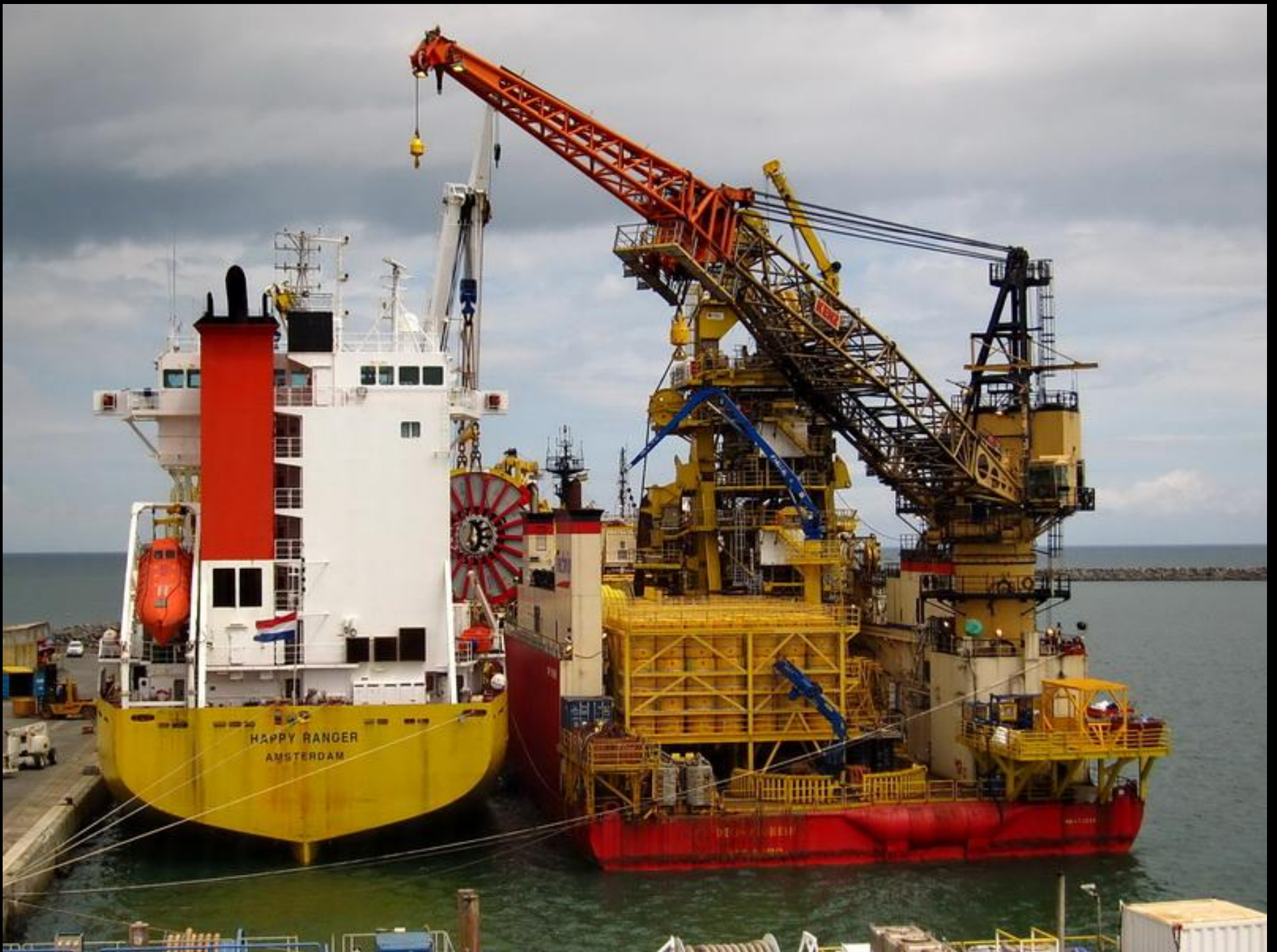
A reel of pipe weighing over 100 tons is being loaded onto Technip's Deep Pioneer to be laid in the Jubilee Field.
