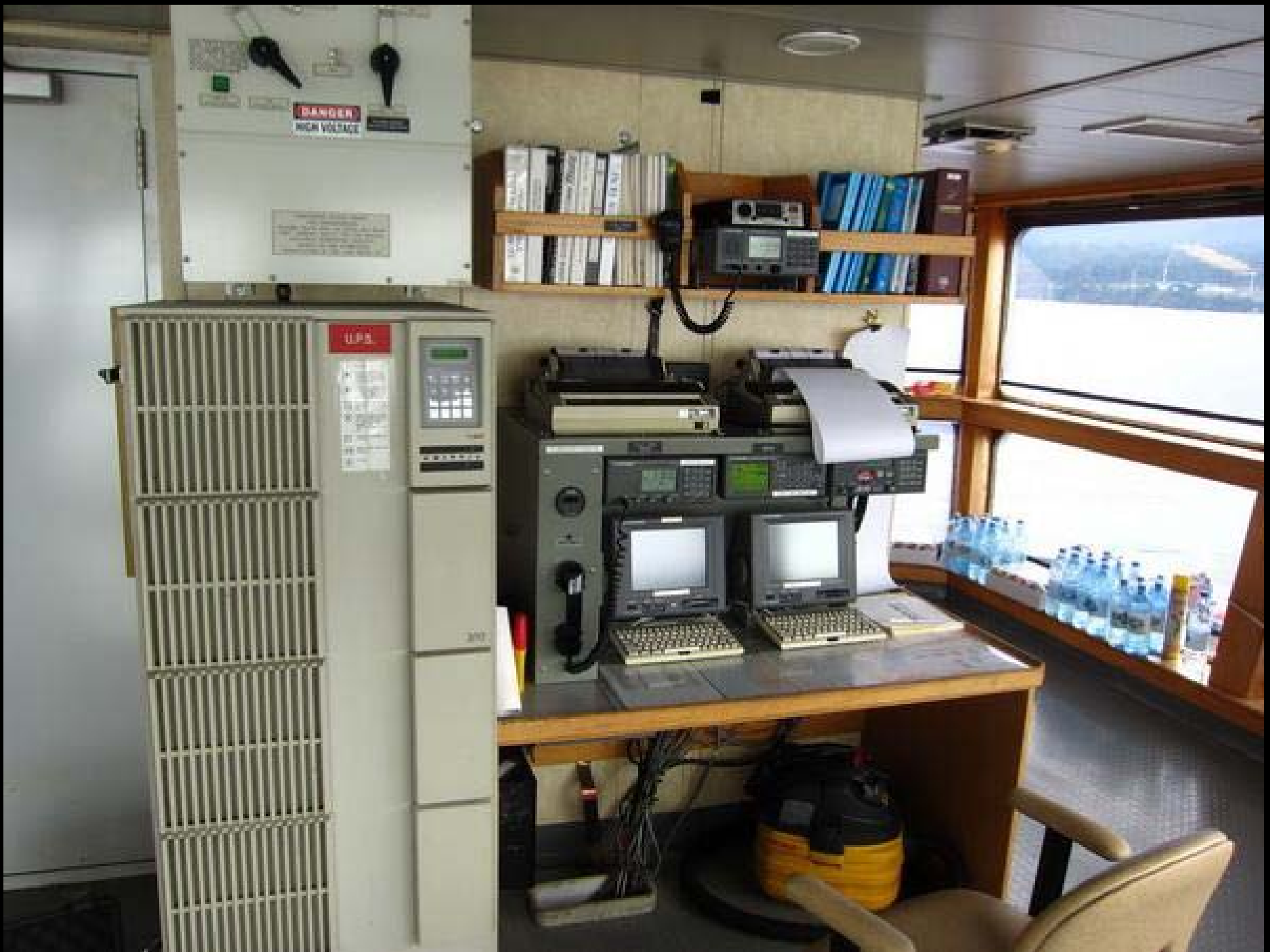
All large vessels are required to have a GMDSS station. The unit to the right is ours. The unit to the left is the UPS (battery backup) for the DP system and other critical electronics.
